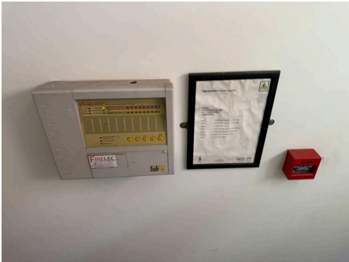
Fire and smoke detection system
