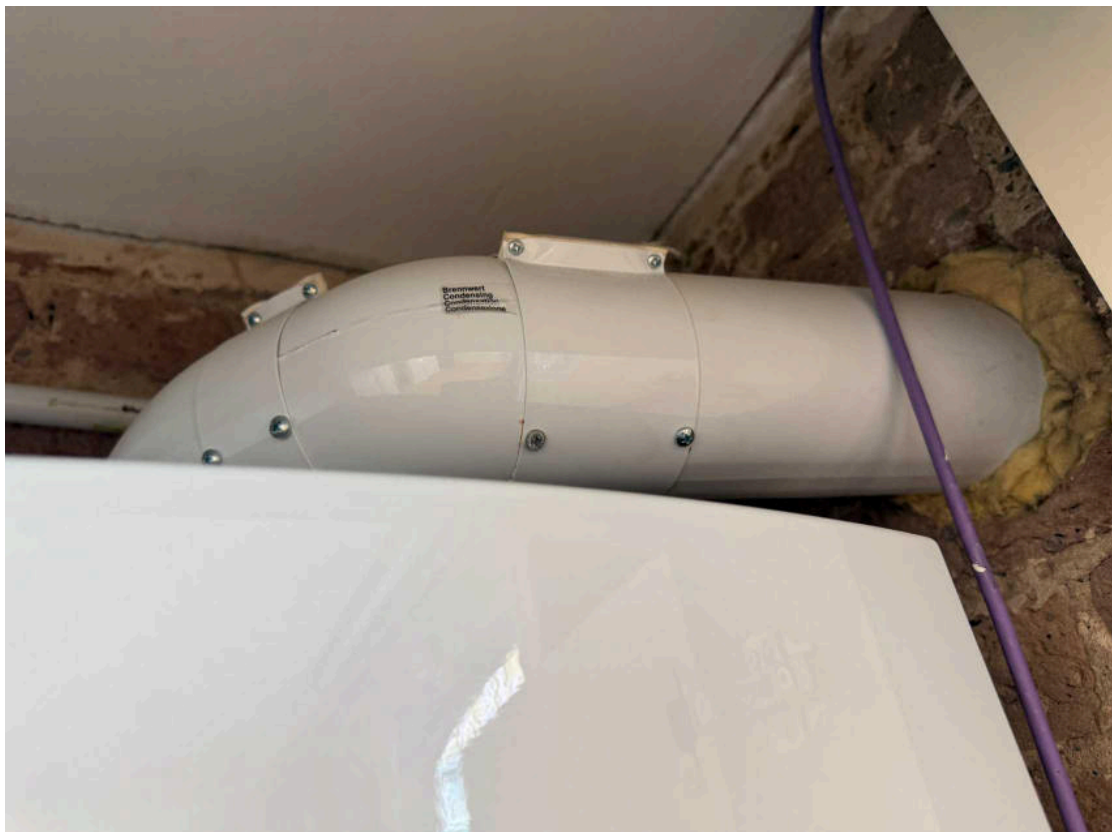
Central heating boiler flue
