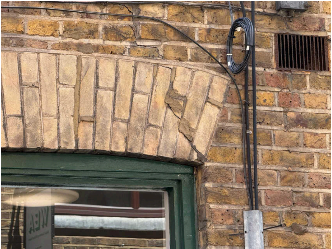
Crack on the comunal door brick arch lintel
