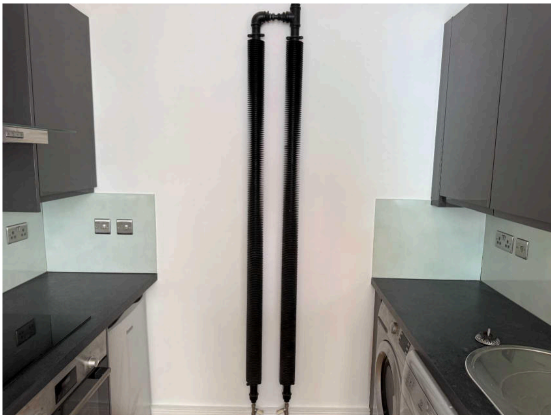
Central heating radiator
