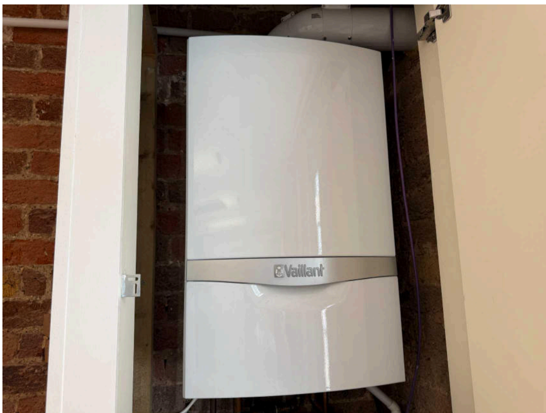
Central heating boiler
