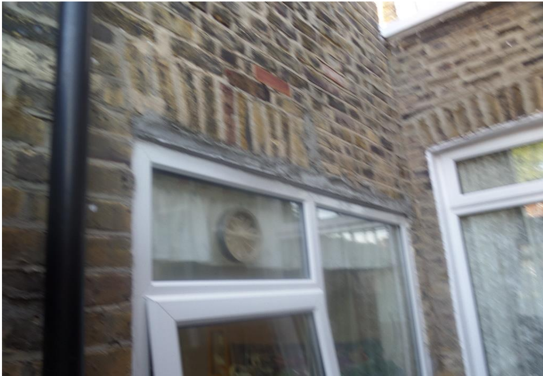
Distortion on the flank wall and lintel over the window
