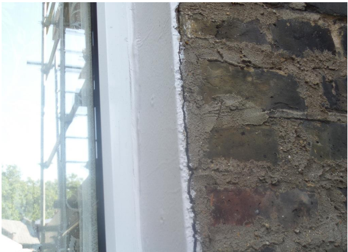
Cracks on reveal
