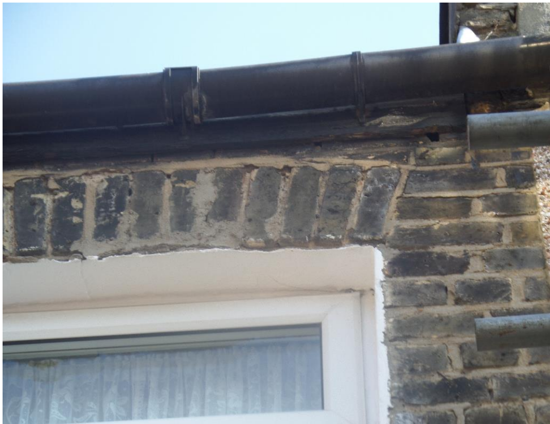
Distortion on brick arch lintel
