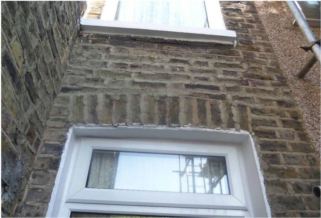
Distortion on the rear wall
